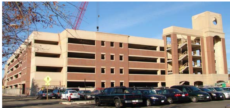
The new Burke Centre Garage, shown here under construction, was opened for VRE parking on Monday, June 2, 2008.
