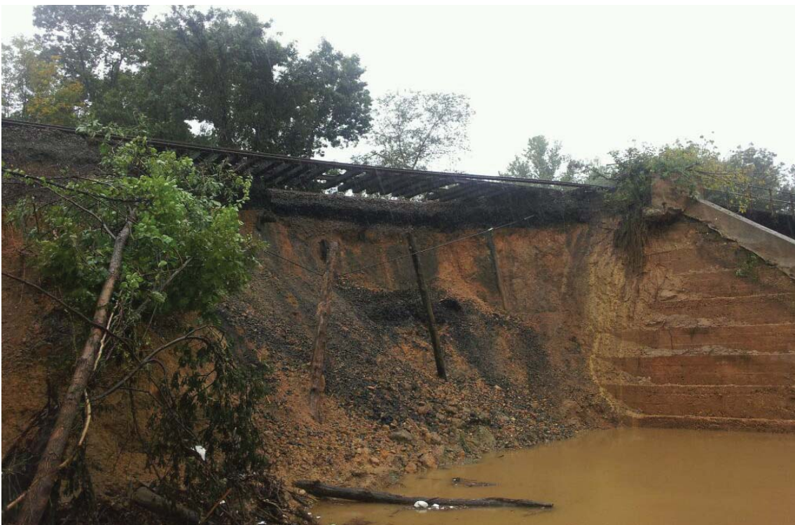
The photo above shows the washout near Franconia/Springfield that caused train delays and service cancellations on Sept 8th and 9th. The washout was spotted by one of our locomotive engineers. Thanks to the flash flood related speed restrictions, he was able to stop the train quickly and safely before reaching the washout.
