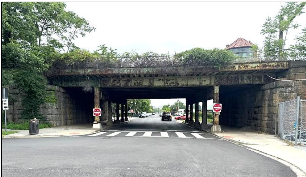
Photo 12: The 2 nd Street Bridge from the intersection with E Street SW, facing north. The top of the 2 nd Street SW Signal Tower is visible above the bridge at right (VHB 2024).
