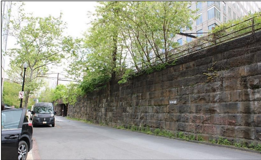
Photo 10. The rusticated stone retaining wall along the south side of Virginia Avenue SW; bridge over 4th Street SW visible in background, facing southeast (VHB 2024).
