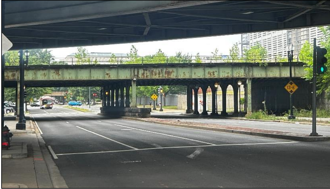
Photo 11. View of the South Capitol Street SW Bridge as viewed from below the I-695 overpasses, facing north (VHB 2024).
