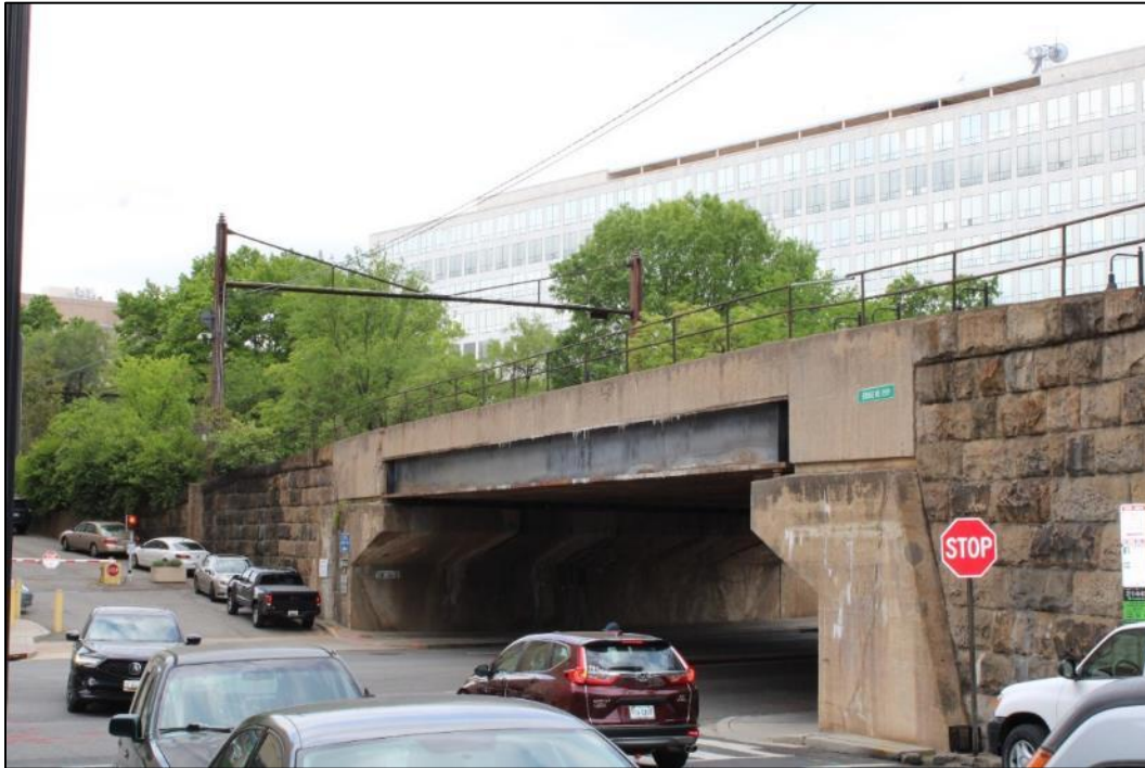
Photo 22. View of the south side of the 7 th Street Bridge with rusticated stone retaining wall on either end, facing northwest (VHB 2024).
