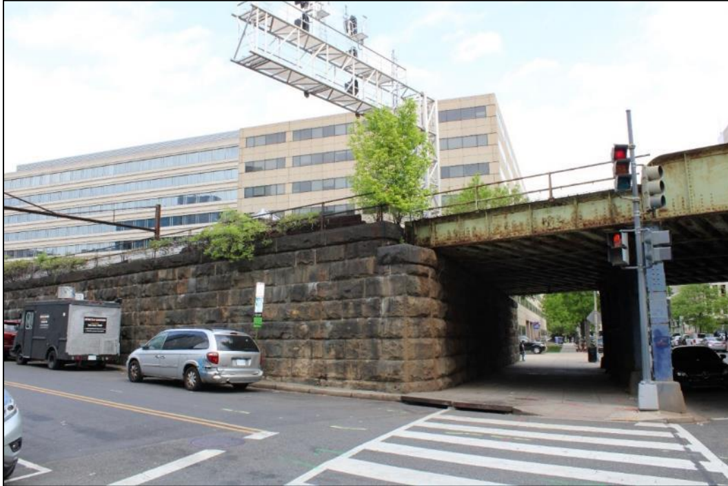
Photo 1. Rusticated stone retaining wall (left) and original steel bridge crossing over 6 th Street SW (right), facing northwest (VHB 2024).
