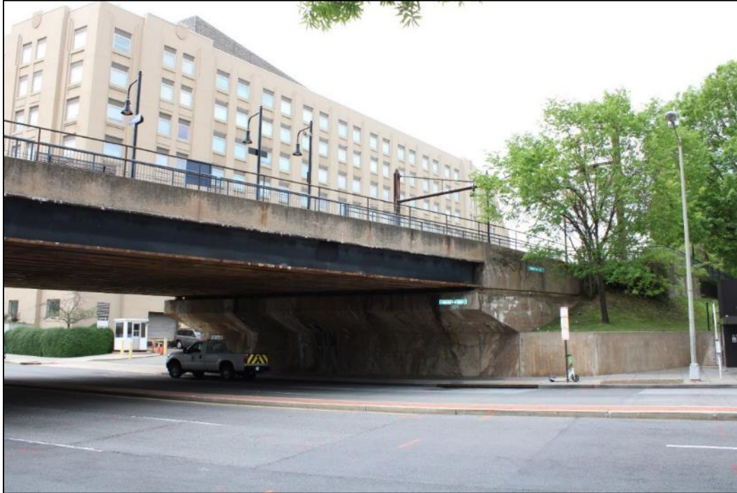
Photo 24. View of the north side of the 7 th Street Bridge, facing southwest (VHB 2024).
