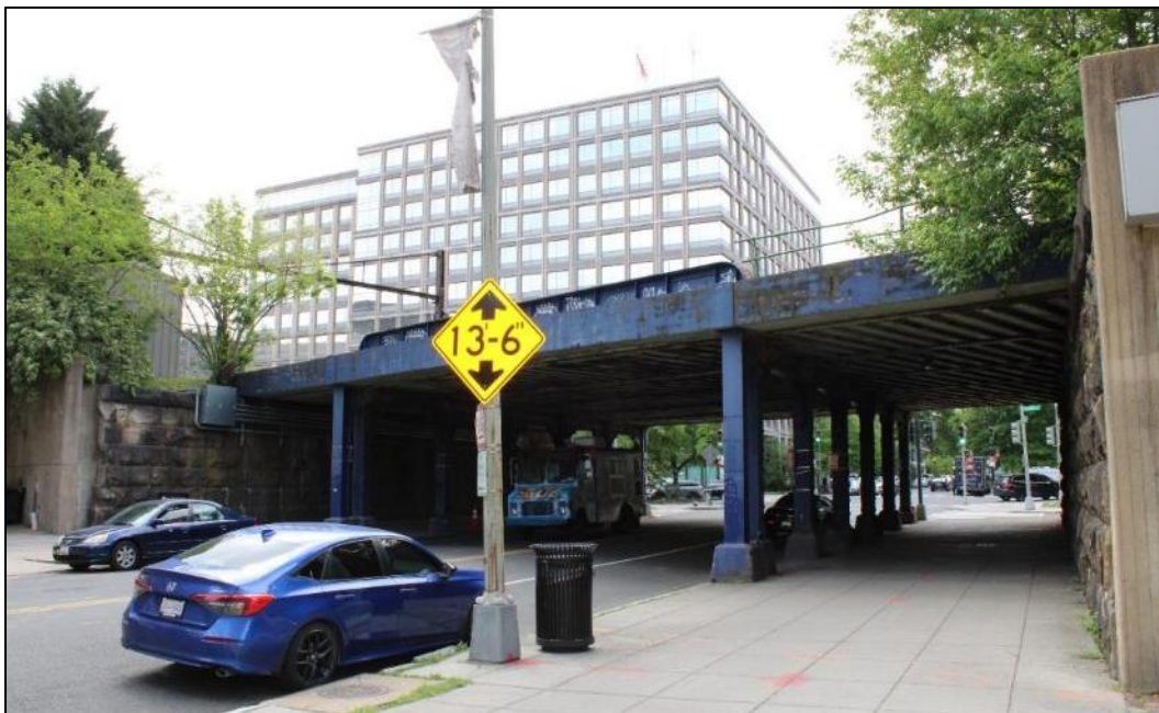
Photo 16. View of the north side of the 6 th Street Bridge near the entrance to the Virginia Rail Express L'Enfant Station, facing southwest (VHB 2024).
