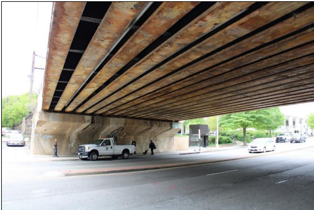
Photo 25. View of the substructure of the 7 th Street Bridge, facing northwest (VHB 2024).
