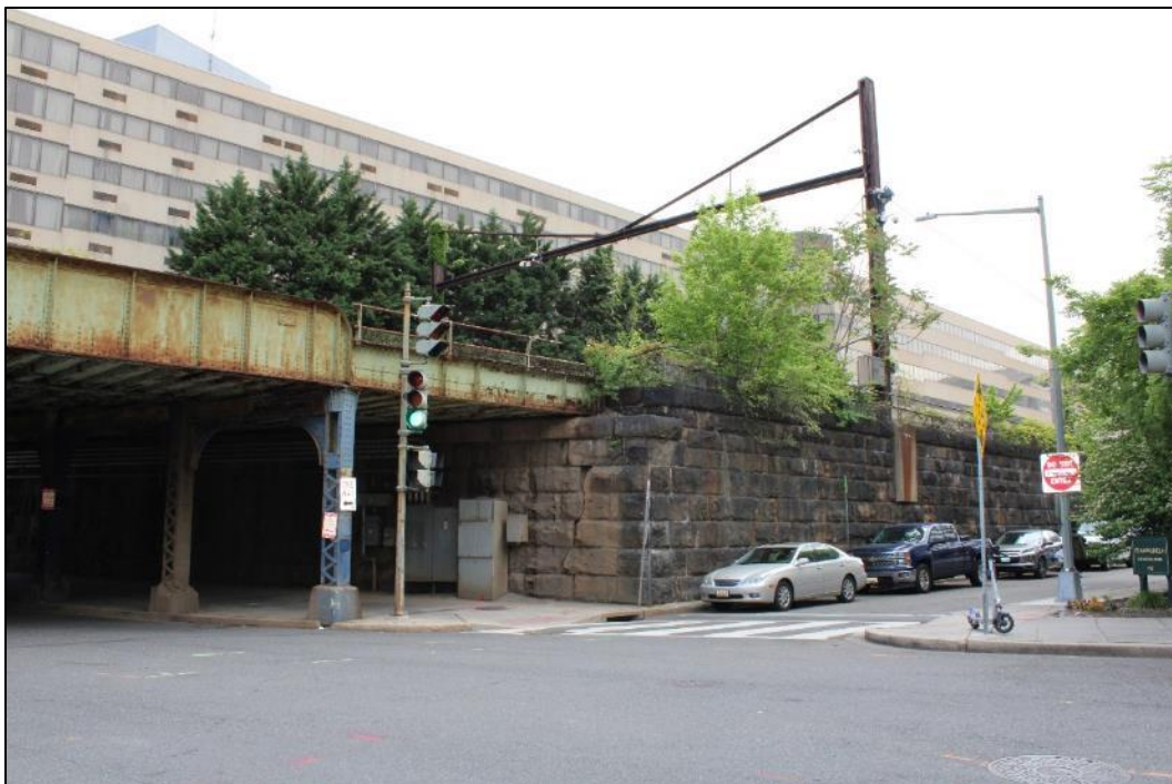
Photo 2: The 6 th Street Bridge, a catenary pole is visible at center right, facing northeast (VHB 2024).
