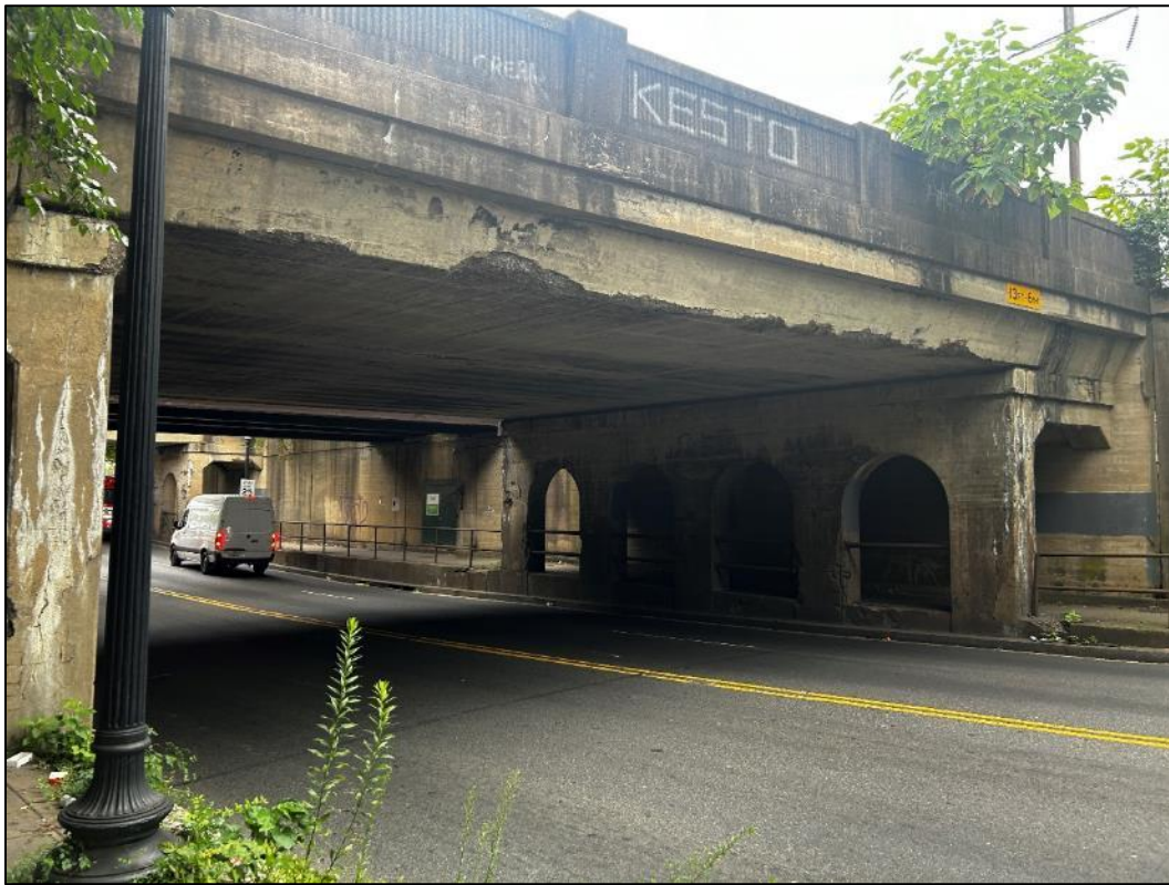
Photo 4: The circa 1915 concrete bridge carrying the railroad over Eastern Avenue NE, facing southeast (VHB 2024).
