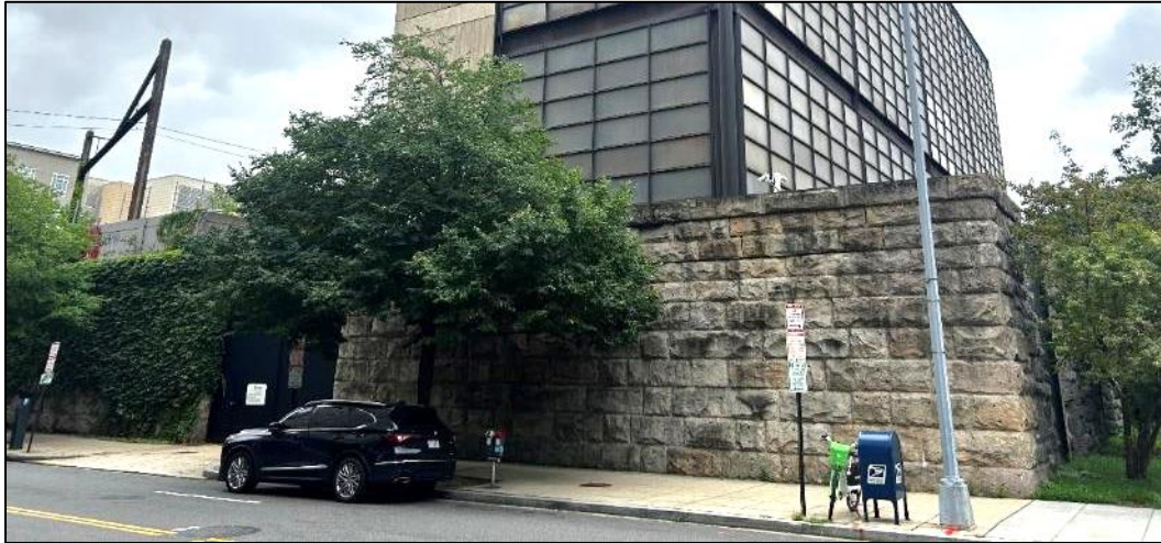
Photo 20: The rusticated stone wall enclosure at 3rd and E Streets SW, facing southeast (VHB 2024).
