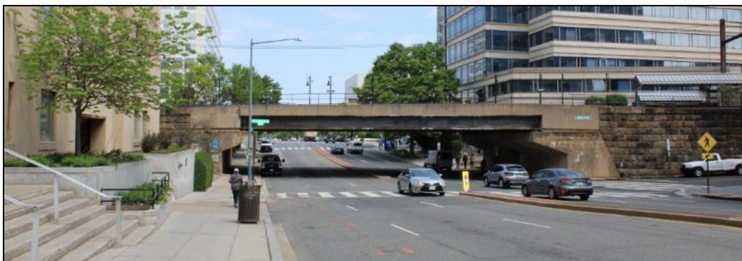
Photo 21. View of the south side of the 7 th Street Bridge, facing north (VHB 2024).
