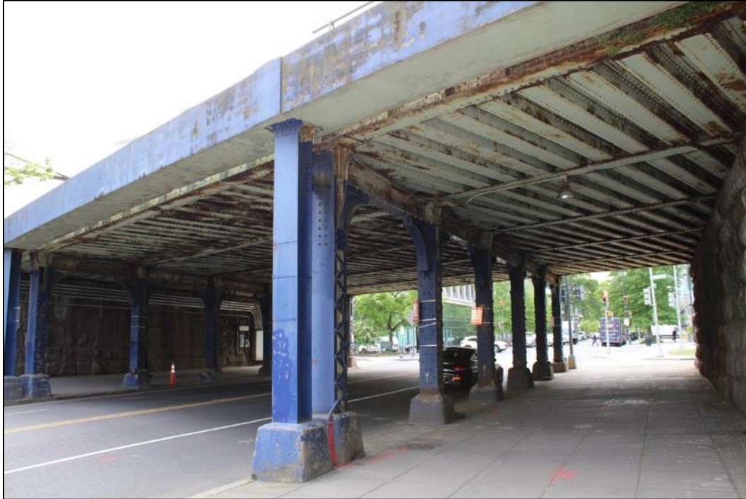
Photo 17. View of the substructure of the 6 th Street Bridge, facing southeast (VHB 2024).
