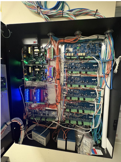
PANEL 2: SERVER ROOM
